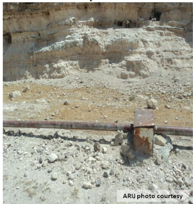
Photo 3: The water line which supply the Bedouin community of Al Khan al Ahmar
